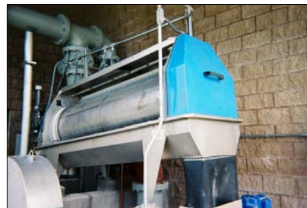
SCREENING: PROTECTS THE DOWNSTREAM MEMBRANES FROM DAMAGE
